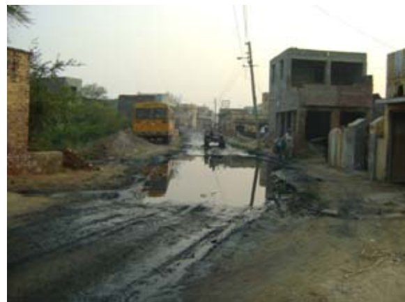
Stagnation of waste water and rain water due to poor drainage
