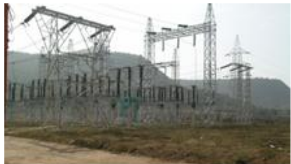
133 KV Sub-Station Gwalior
