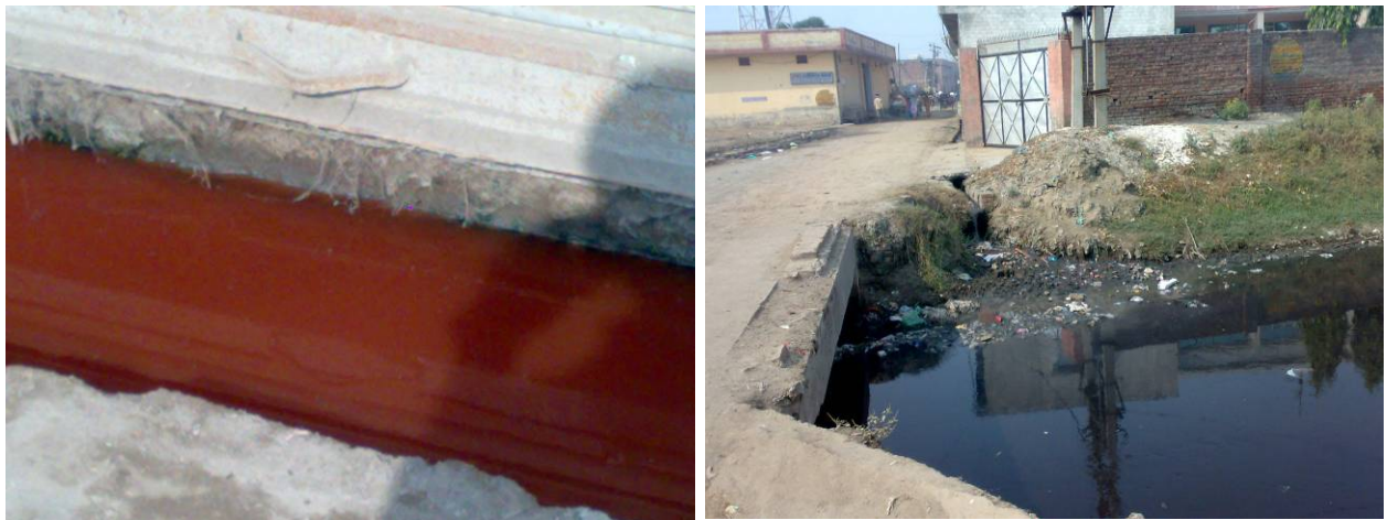
Photograph 1 and 2: Condition of Open Drains in Panipat Old Industrial Area
